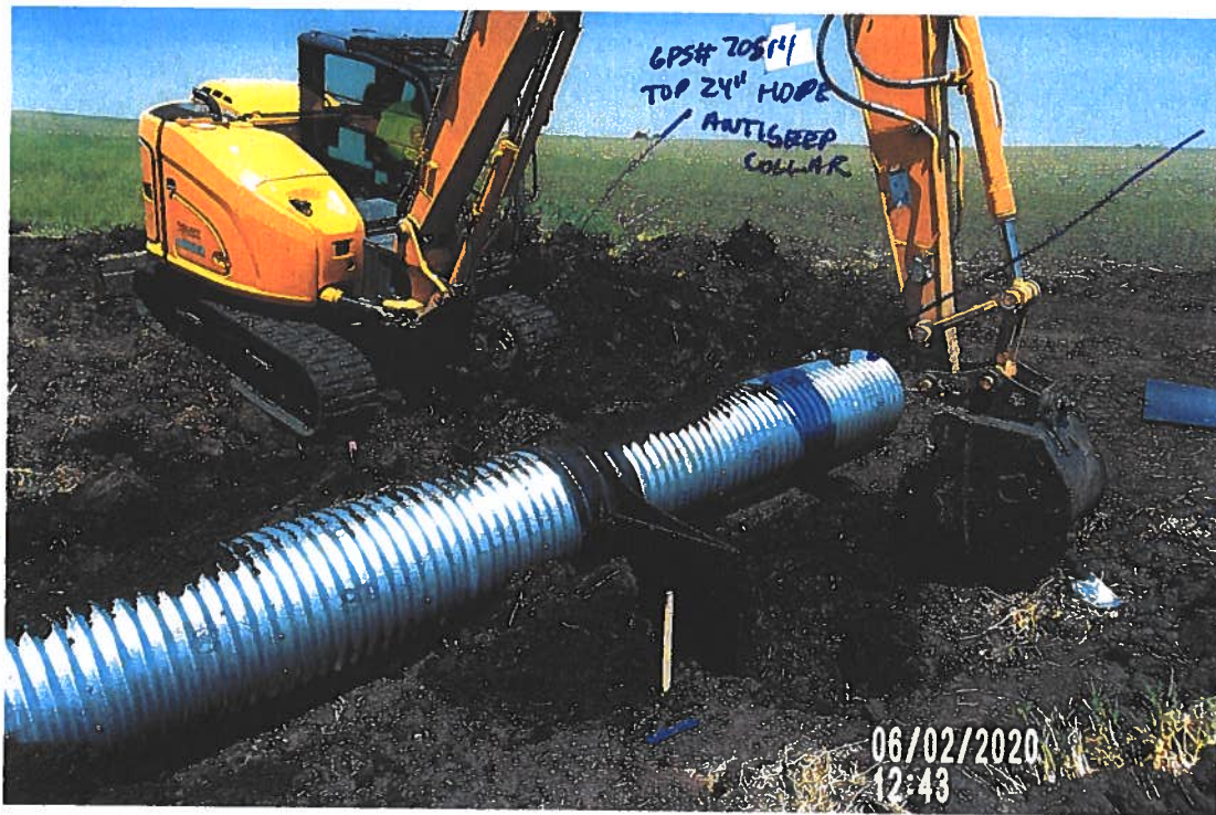
PICTURE# 3633 IS LOOKING NW SHOWING 24" HDPE ANTISEEP COLLAR IN PLACE WITH 2 BANDS AND 5 BOLTS FASTENING LOWER ANTISEEP AND PARTIAL UPPER ANTISEEP HDPE COLLAR ONE EAST SIDE
