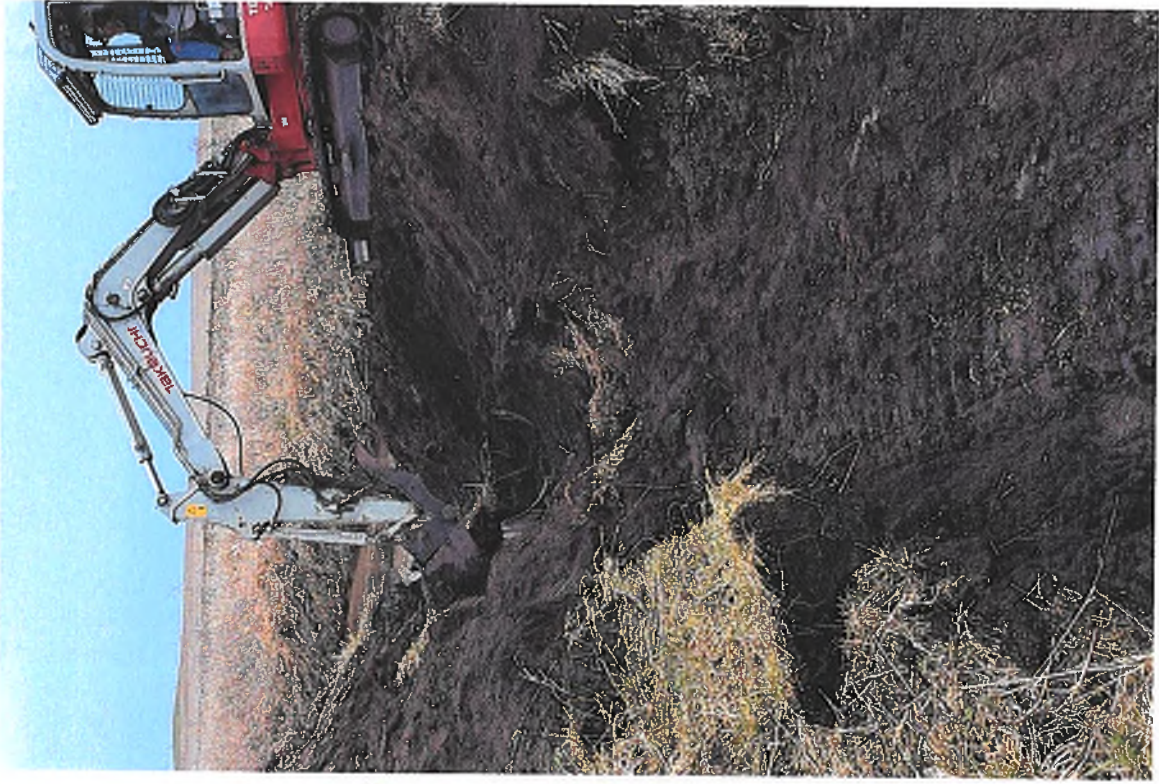
PICTURE # 16 IS LOOKING SOUTH SHOWING EXCAVATOR DIGGING TO REMOVE ANTI SEEP COLLAR.
