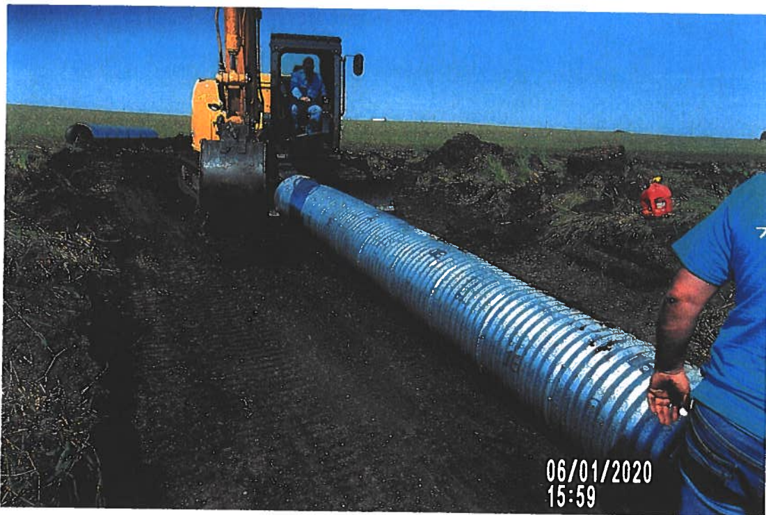
PICTURE #3622 IS LOOKING NE SHOWING CREW PUSHING IN NEW CMP AFTER BOTTOM OF TRENCH GRADED AND JUMPING JACK COMPACTED.
