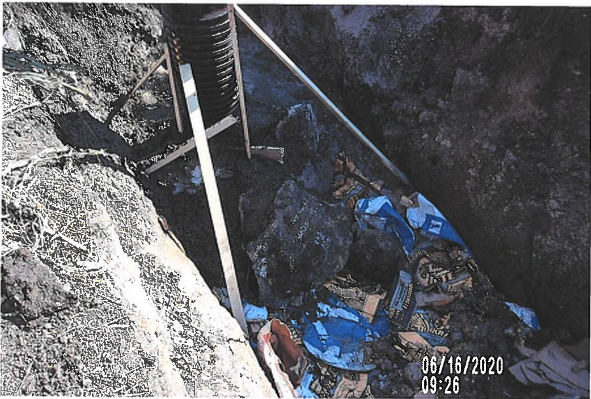
PICTURE # 3767 IS LOOKING NE SHOWING OLD CONCRETE CHUNKS CONCRETED IN TO SUPPORT 8" SW HOPE PERF TILE FOR 8" HICKEN BOTTOM INTAKE.
