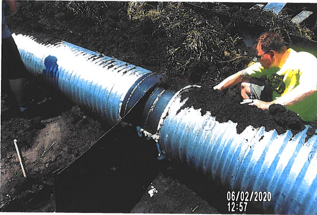
PICTURE # 3636 IS LOOKING EAST SHOWING CREW USING FOAM FILL TO SEAL BETWEEN HDPE ANTISEEP COLLAR AND 24" CMP SURFACE DRAIN, (SUDAS SHOWS SHOULD BE BITUMINOUS MATERIAL)
