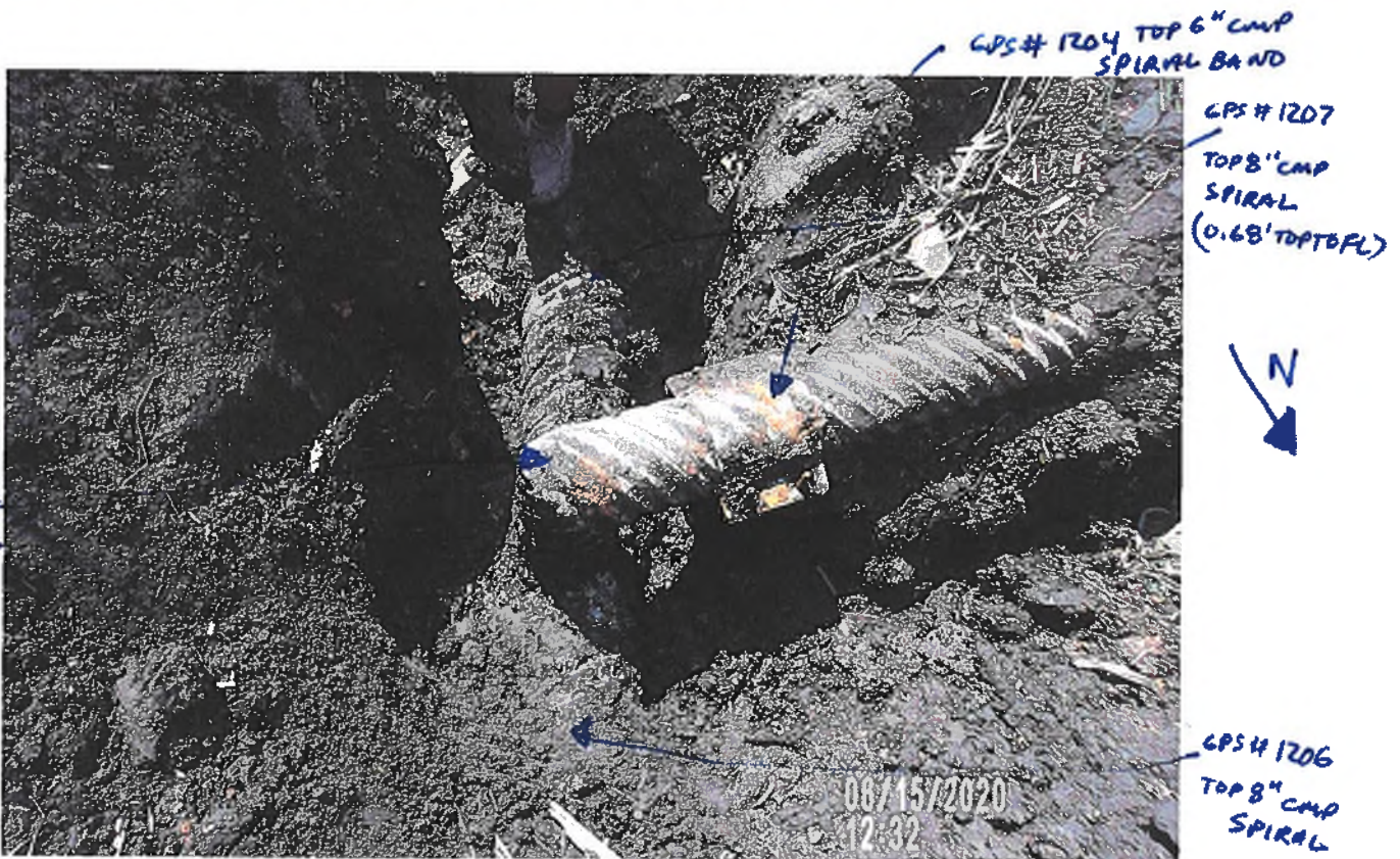
PICTURE # 3749 IS LOOKING SW AT 6" CMP SPIRAL FROM FIELD TIED INTO 8" CMP SPIRAL FROM BEEHIVE INTAKE AFTER BEEHIVE INTAKE HAS BEEN REMOVED
