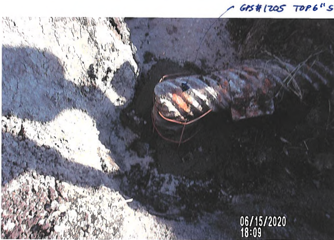
PICTURE # 3762 IS LOOKING SOUTH SHOWING 1.0' X 2.0' 6" X 6" WIRE MESH AROUND 6" TO 8" CMP SPIRAL CONNECTION BEFORE CONCRETE POURED.
