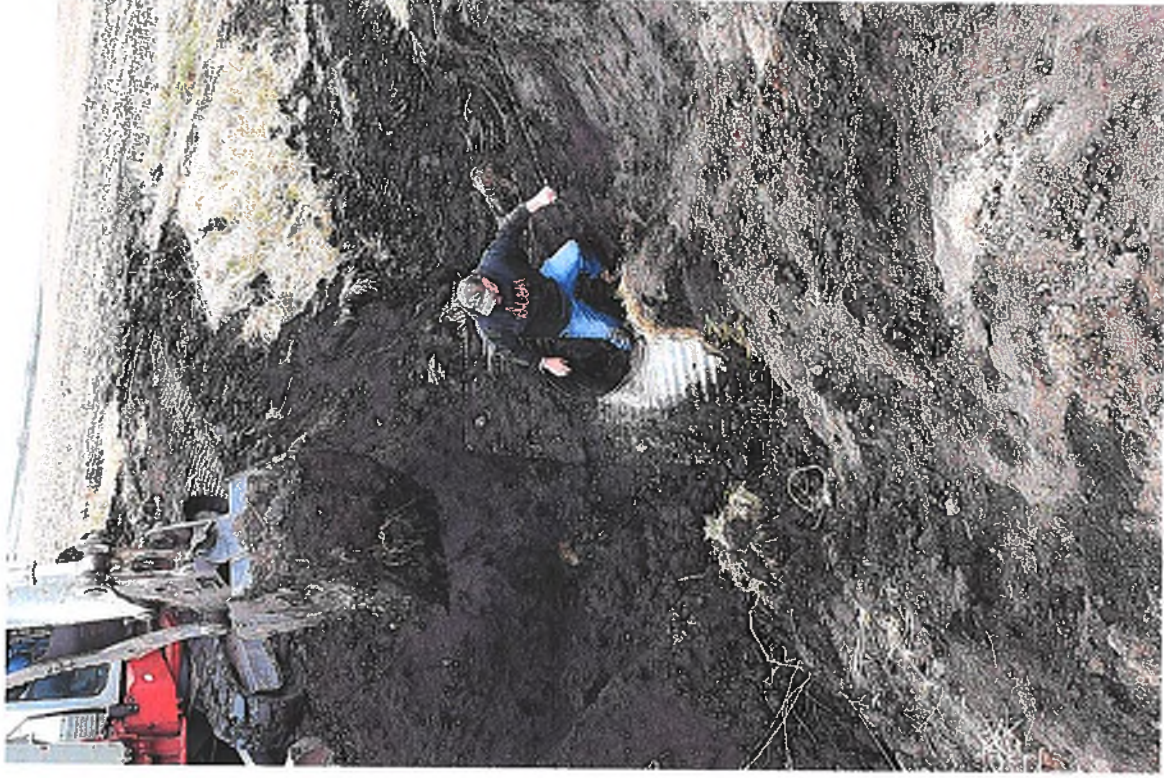
PICTURE # 17 IS LOOKING NW SHOWING CREW REMOVING EXISTING METAL ANTI SEEP COLLAR
