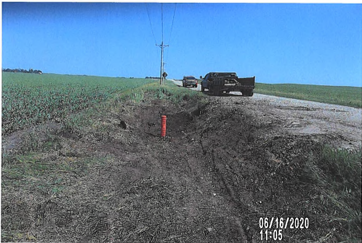
PICTURE # 3772 IS LOOKING NORTH SHOWING DITCH GRADED TO NEW 8" HICKEN BOTTOM INTAKE & SHOWS DITCH GRADED FROM 36" R/P TO NEW 8" HICKEN BOTTOM
