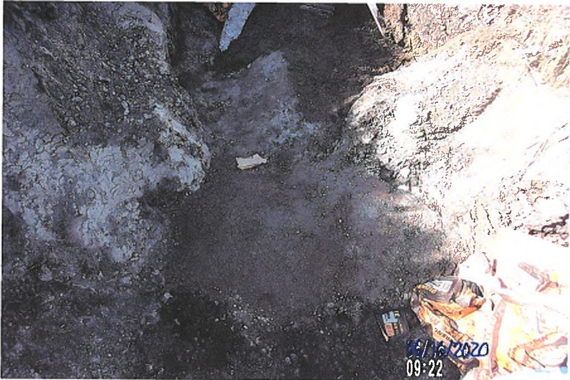
PICTURE # 3766 IS LOOKING SW SHOWING CONCRETE COLLAR FINISHED AROUND 6" 90° CMP SPIRAL ELBOW TO 8" CMP SPIRAL TO 8" HOPE SW PERF TILE.
