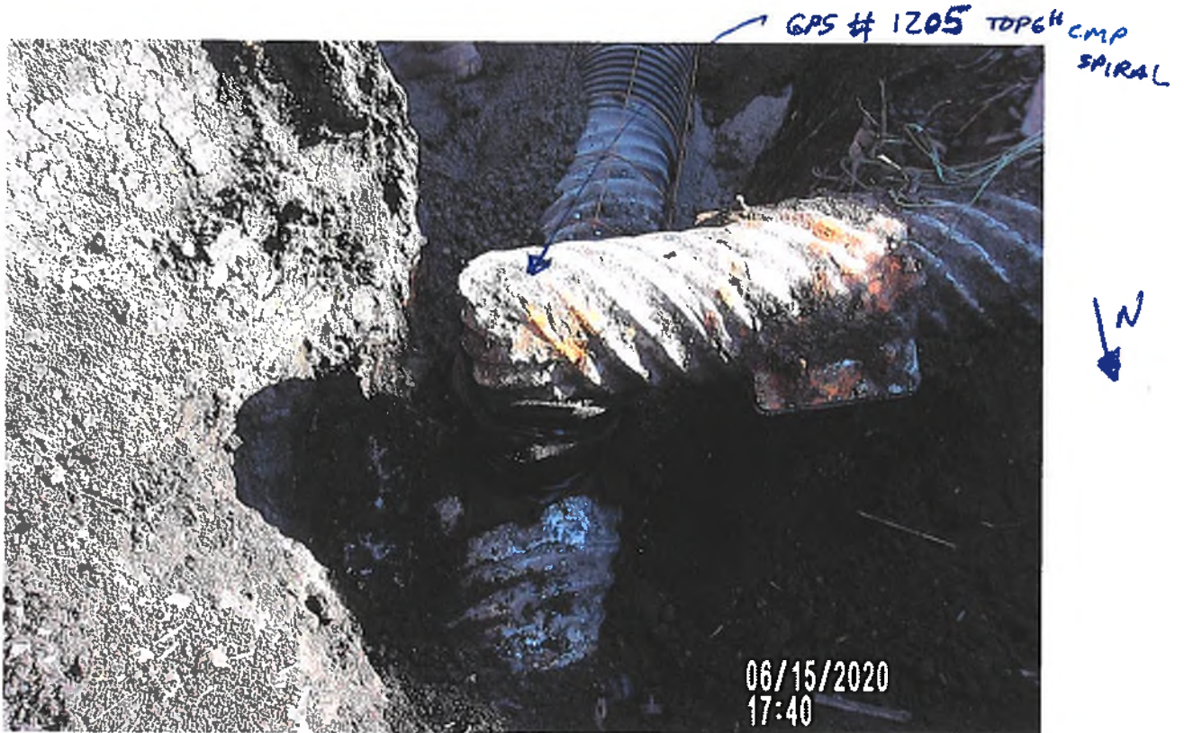
PICTURE # 3759 IS LOOKING SW SHOWING 6" 90° CMP SPIRAL TIE IN INTO 8" CMP SPIRAL WRAPPED WITH FABRIC & TILE TAPED BEFORE CONCRETE COLLAR POURED,
