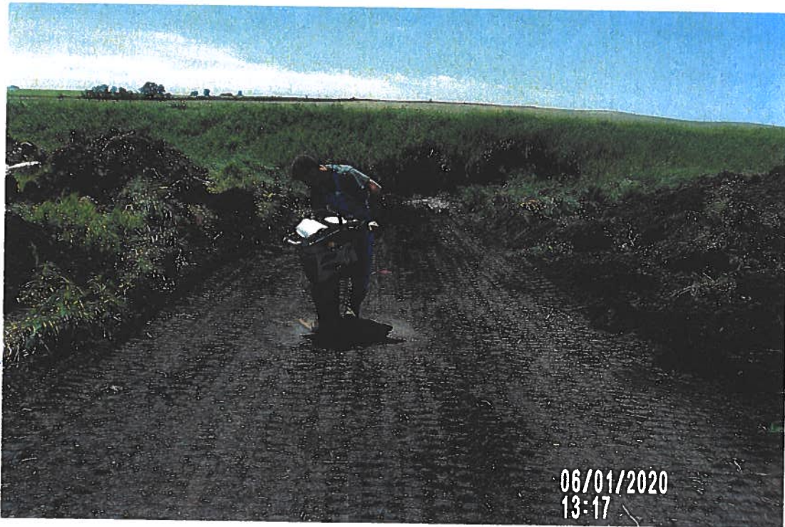
PICTURE# 3620 IS LOOKING SW SHOWING CREW JUMPING JACK COMPACTING BOTTOM OF TRENCH FOR NEW 24" CMP SURFACE DRAIN
