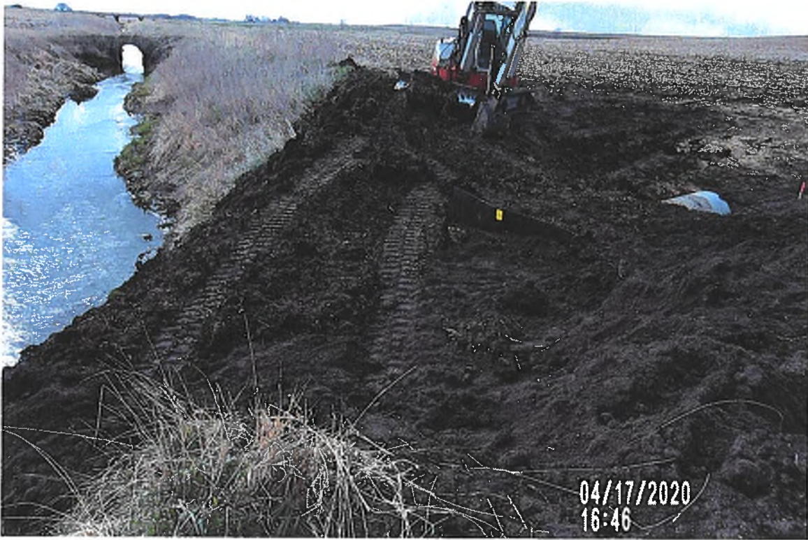
PICTURE #3394 IS LOOKING NW SHOWING CREW BACKFILLING DRAINAGE DITCH BANK AROUND 36" CMP & HDPE ANTISEEP COLLAR
