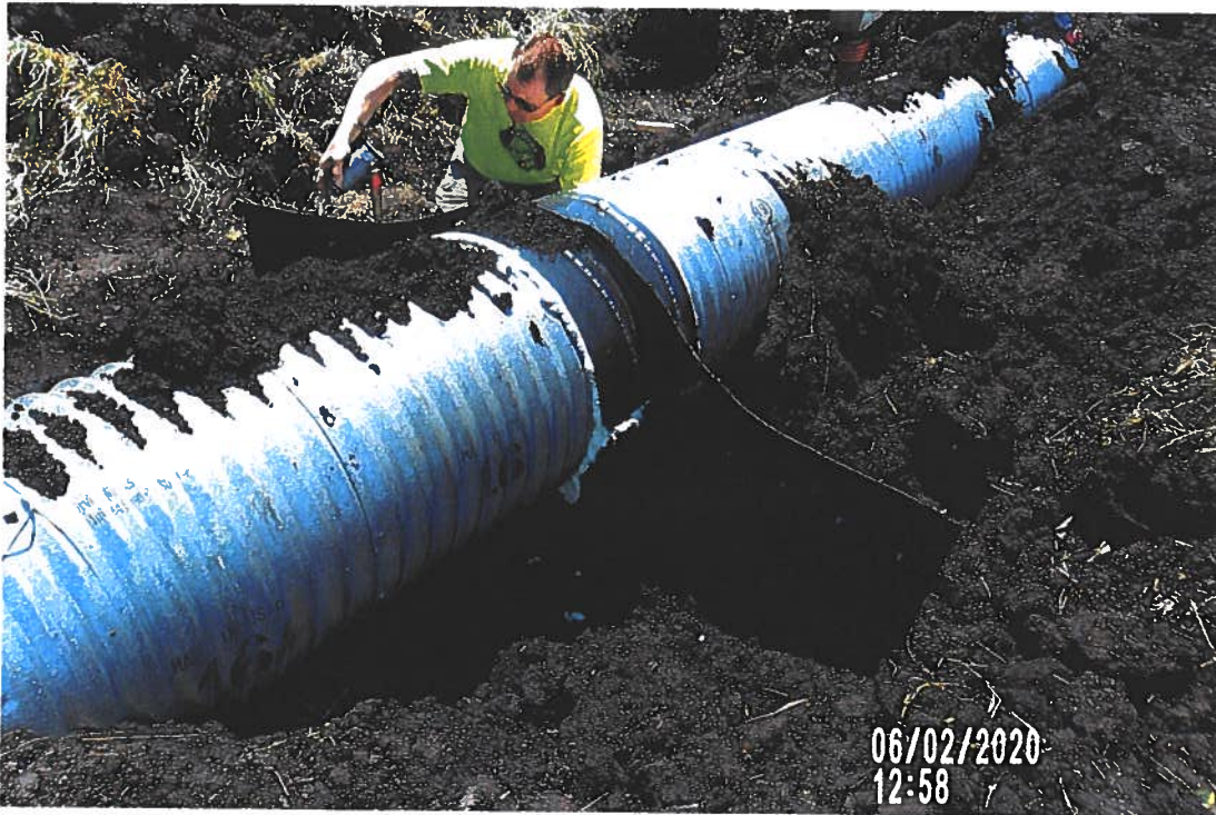
PICTURE # 3637 IS LOOKING SE SHOWING CREW USING FOAM FILL TO SEAL BETWEEN HDPE ANTISEEP COLLAR AND 24" CMP SURFACE DRAIN. (SUDAS SHOWS SHOULD BE BITUMINOUS MATERIAL)
