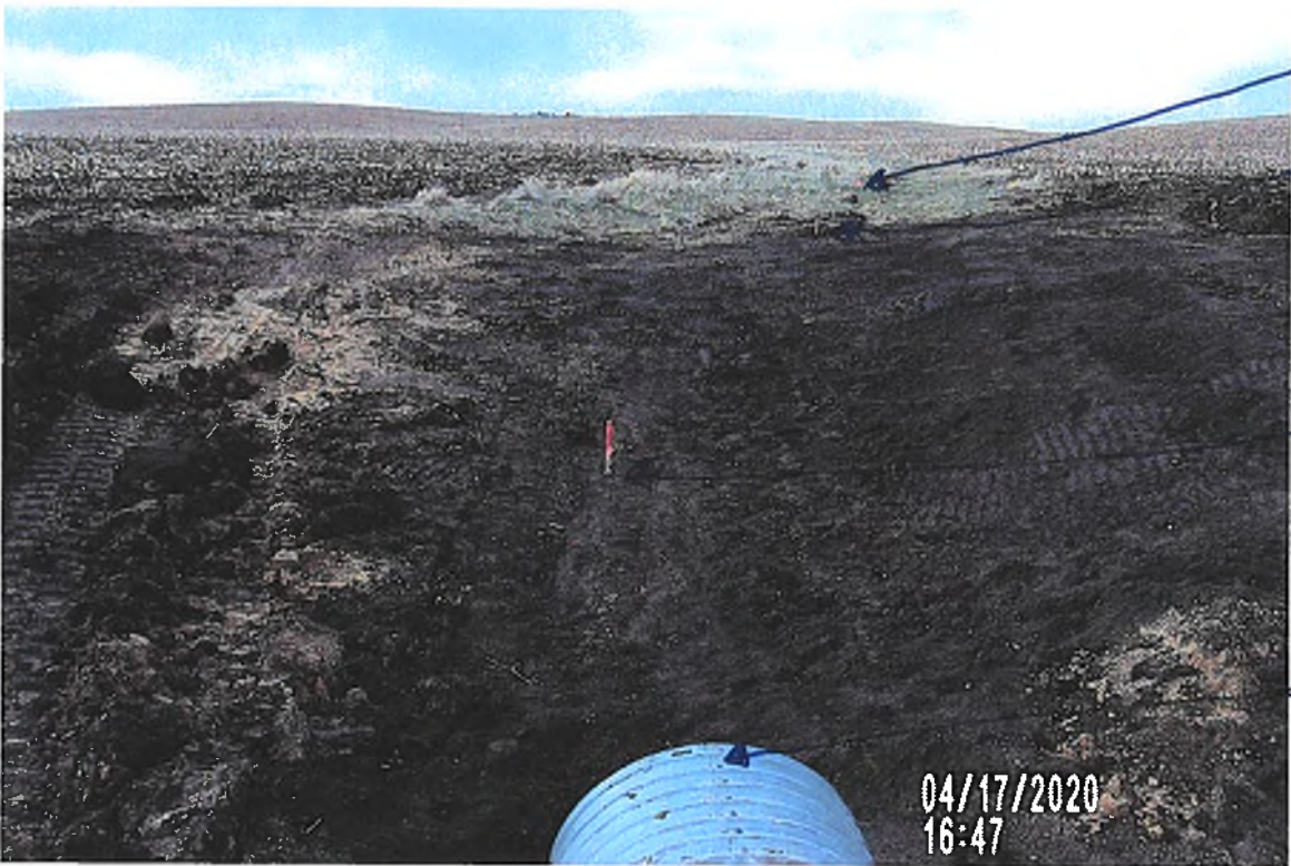
PICTURE #3395 IS LOOKING NW SHOWING GRASS WATERWAY ROUGH GRADED. OBSERVER SET SOME GRADE STAKES FOR CONTRACTOR.
