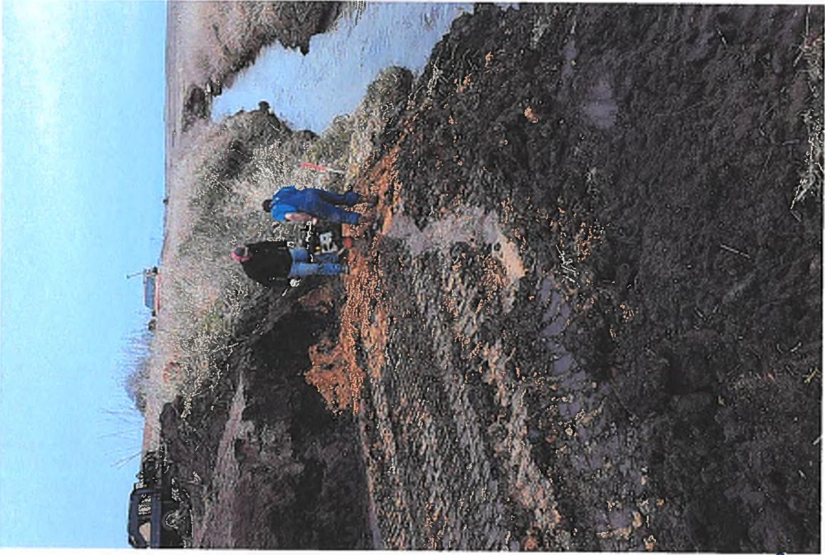
PICTURE #20 IS LOOKING SE SHOWING CREW JUMPING JACK COMPACTING SOUTH END OF TRENCH FOR SURFACE DRAIN PIPE.
