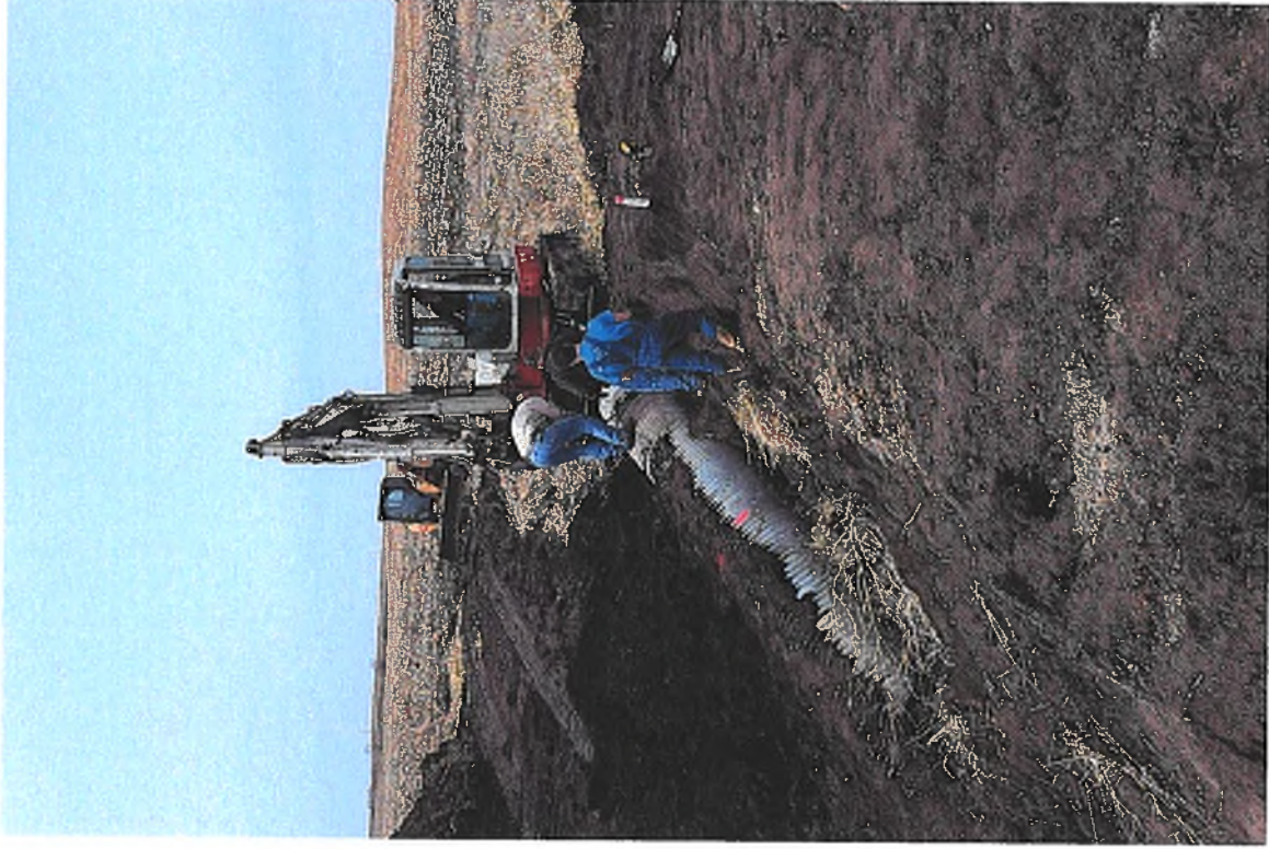
PICTURE #13 IS LOOKING NW SHOWING CREW GETTING READY TO REMOVE 36" CMP SURFACE DRAIN
