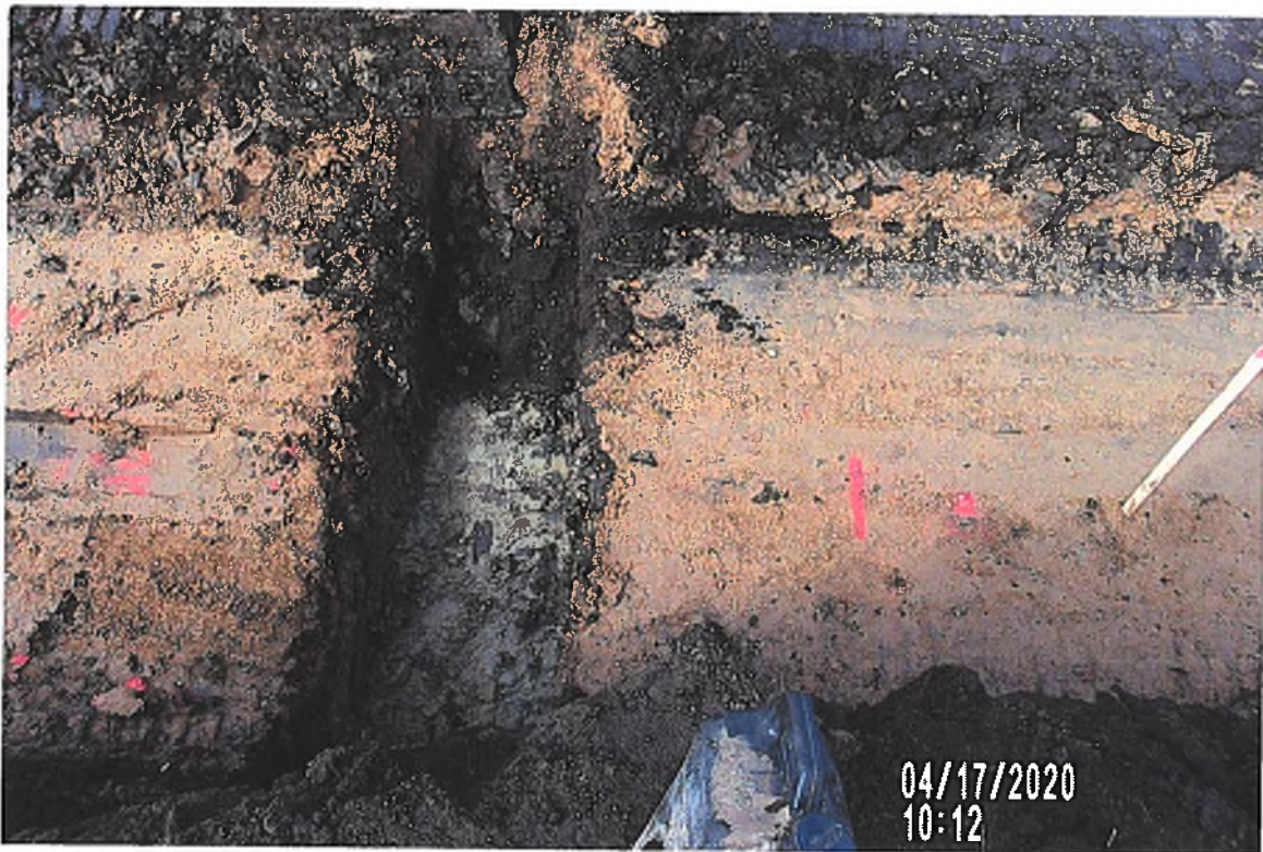
PICTURE # 3372 IS LOOKING SW SHOWING 1.0' X 7.0' WIDE TRENCH FOR ORIGINAL METAL ANTI SEEP COLLAR 7.0' ± SE OF NORTHEND OF CMP SURFACE DRAIN. BOTTOM OF TRENCH IS CLAY.
