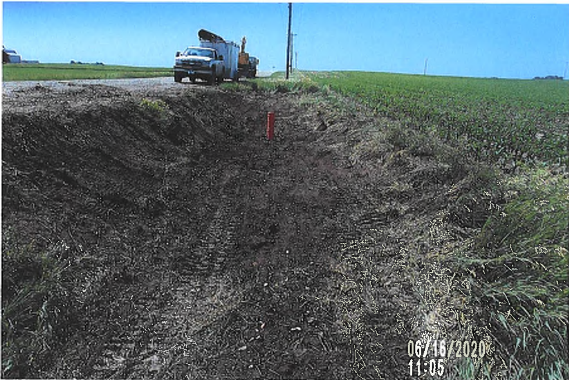
PICTURE # 3771 IS LOOKING SOUTH AT DITCH GRADED TO NEW 8" HICKEN BOTTOM INTAKE.
