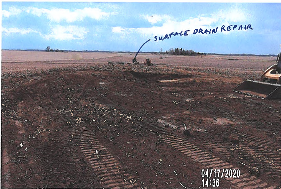
PICTURE # 3389 IS LOOKING SW FROM BORROW AREA TO CMP SURFACE DRAIN REPAIR ABOUT 713.6' TO SW
