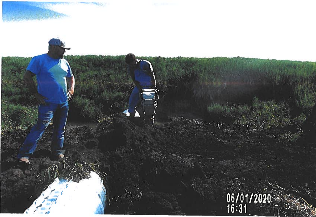
PICTURE # 3625 IS LOOKING SOUTH SHOWING CREW STILL BACKFILLING WITH LOOSE SOIL AND JUMPING JACK COMPACTING SOIL AROUND CMP
